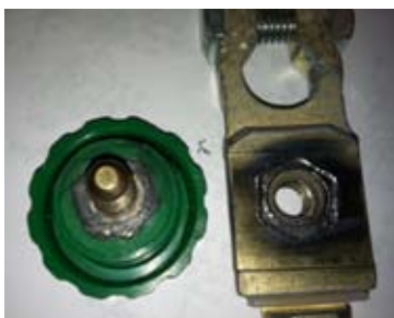
Damaged battery disconnect
