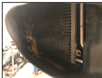
Just beginning the job and seeing leaves and other debris in the radiator ductwork.
