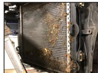
Debris was packed in between the condenser and radiator.
