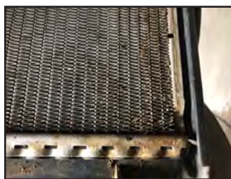
After cleaning you can see the corrosion that has started due to the wet debris.
